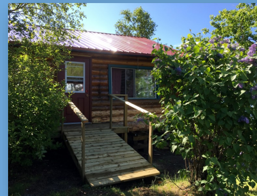
New door and ramp for the Main Lodge, and it is now level
