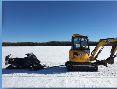
The little Backhoe made the 7 hour trek across the ice & the portage! It will make work easier!
